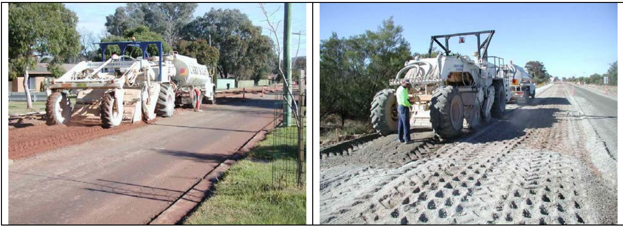
Figure 2 DPP being used in urban and rural sites using conventional insitu stabilisation equipment.
